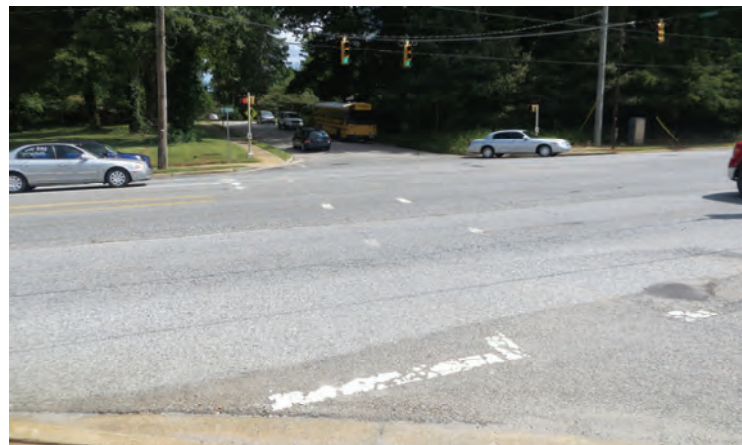
Faded crosswalk at the Cherry Rd./Richmond Dr. intersection
