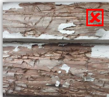
SIDING DAMAGED BY HIGH PRESSURE WATER CLEANING METHOD
