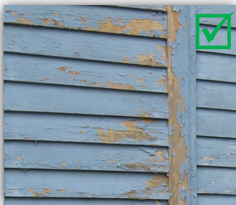
SIDING IN NEED OF SCRAPING AND REPAINTING
